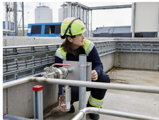
Tapping oil at the Skive plant in Denmark
